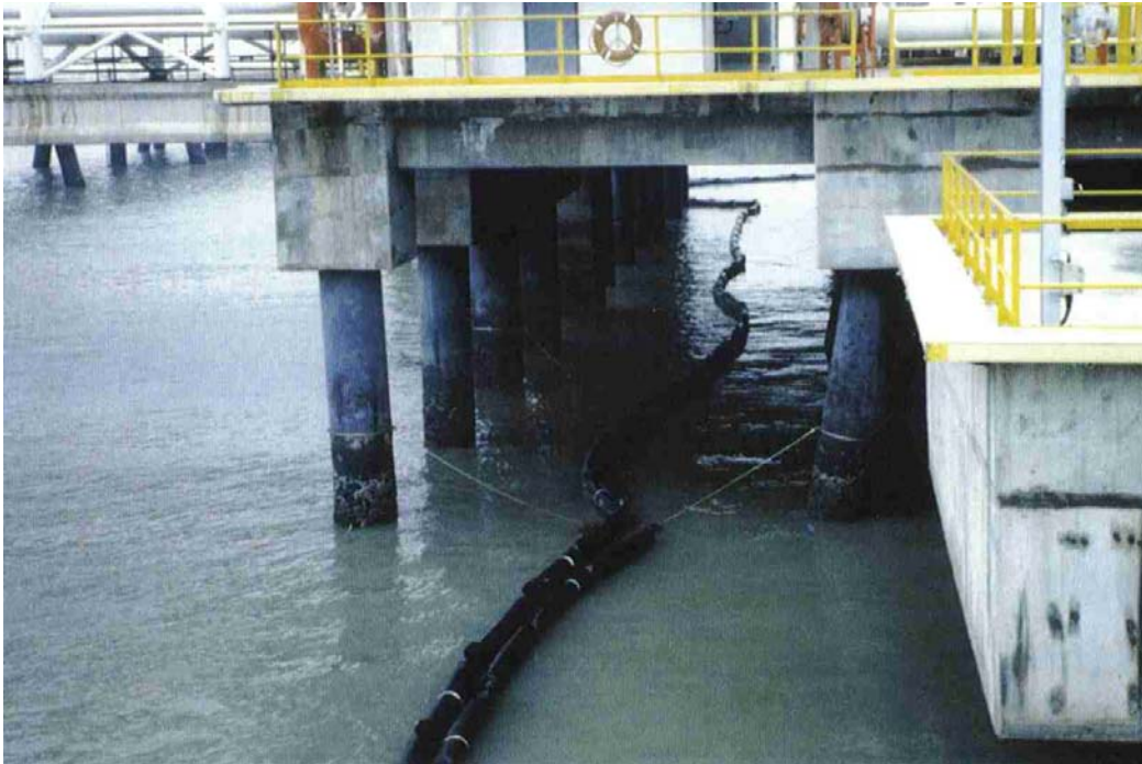
Permanent Boom tethered under pier
