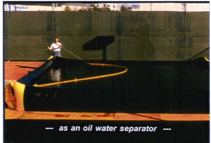
KepBerm systems are used for outdoor storage of hazardous chemicals ---
